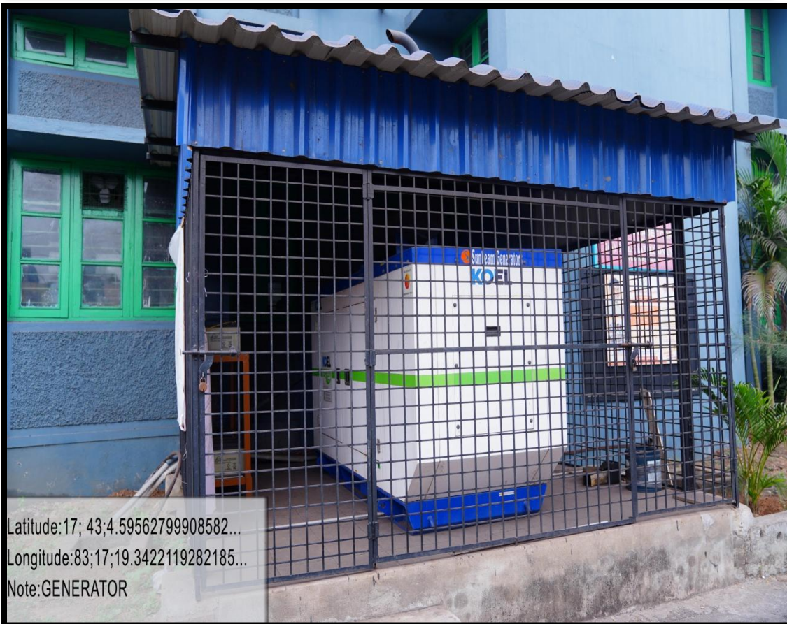
Latitude:17; 43;4.14778804083468... Longitude:83; 17;18.4647119875299... Note:GENERATOR 2
